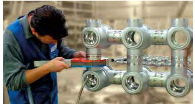
Figure 1. Installation in a food and beverage plant with an orbital welding head. The workpieces must be properly positioned to avoid misalignment.
