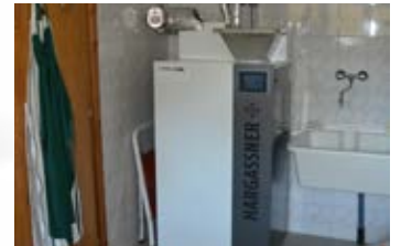
Heizraumvarianten / Various Heating rooms
