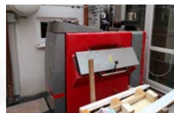
Heizraumvarianten / Various Heating rooms
