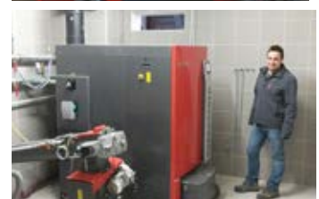
Heizraumvarianten / Various Heating rooms
