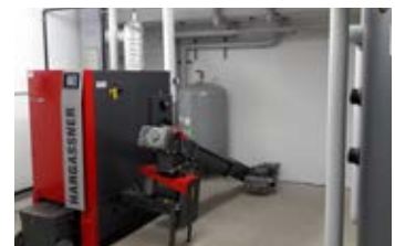
Heizraumvarianten / Various Heating rooms
