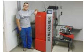
Heizraumvarianten / Various Heating rooms
