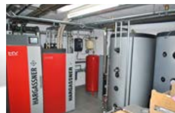
Heizraumvarianten / Various Heating rooms
