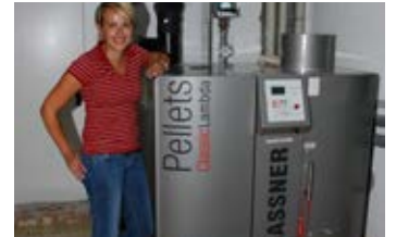
Heizraumvarianten / Various Heating rooms
